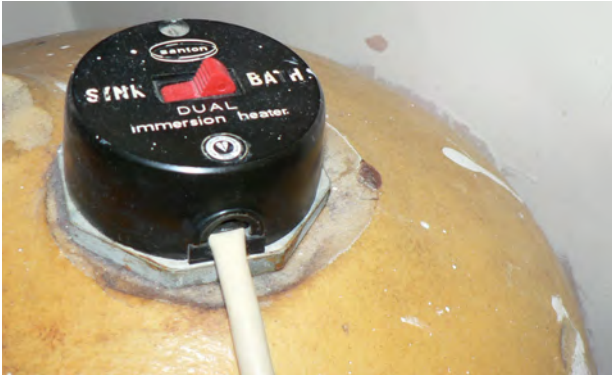
Older immersion heater without thermal cut-out
