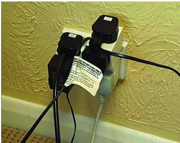
Potentially overloaded socket-outlet
