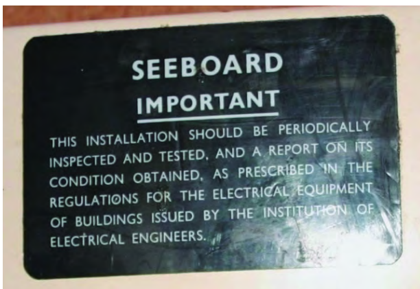
A typical periodic inspection notice for an older installation
