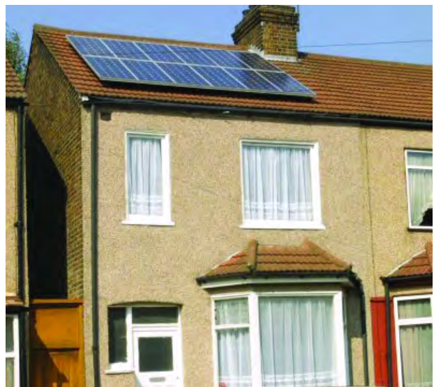
Photovoltaic installation (photo courtesy Energy Saving Trust)
