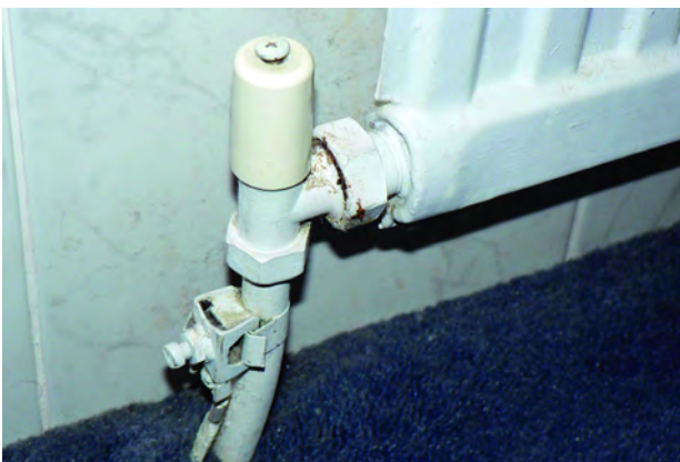
Unmarked bonding conductor
