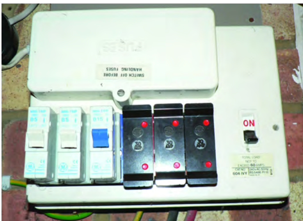
Consumer unit with fuses and circuit-breakers
