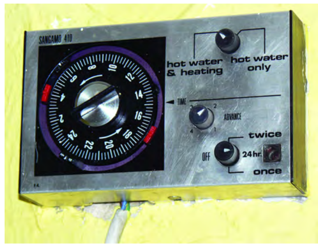
Cable sheath not taken inside enclosure
